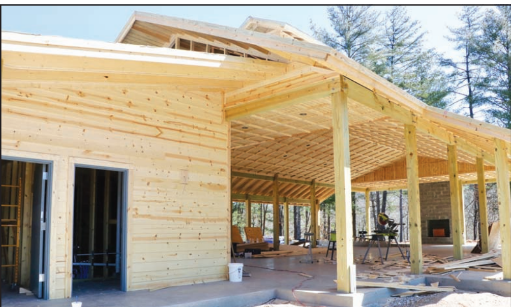
Construction is nearing completion on the brand new pavilion at Meeks Park, which is located adjacent to the baseball fields at the upper part of the park. Photo by Mark Smith
